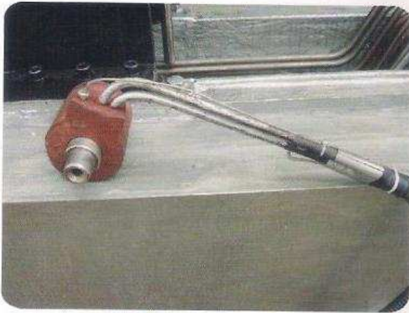
夾具加固：避免因搖動造成斷裂及漏電和短路現象 Jig reinforcement: Avoid break, leakage and short circuit caused by shaking.
